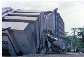
Earthquake-induced damage during 1995 Kobe Earthquake
